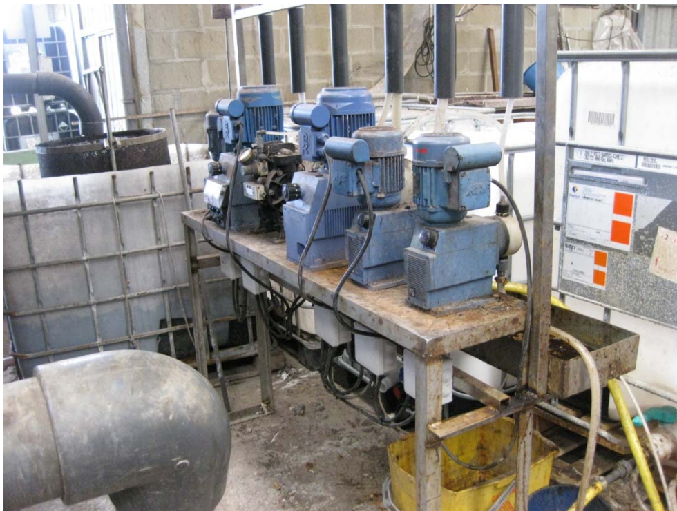
Figure 4. pH regulation addition system on a physical-chemical treatment ETP. (Arteixo. España)
