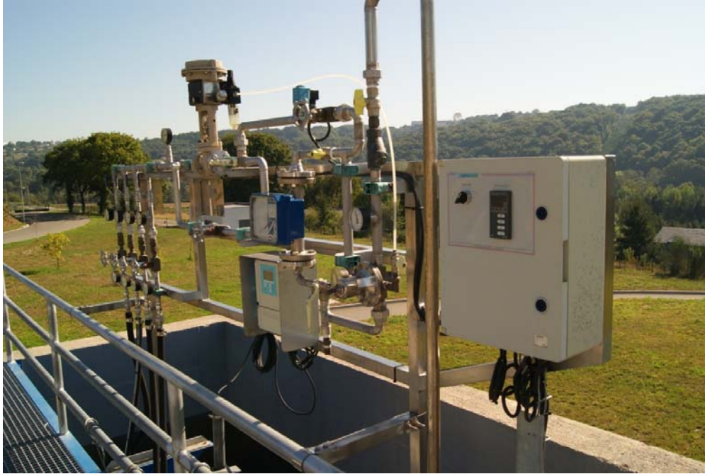
Figure 1. PH regulation system (Drinking water treatment plant -Lugo)
