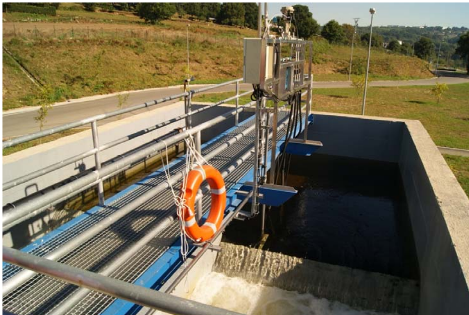
Figure 2. Head pH regulation chamber (Drinking water treatment plant-Lugo)
