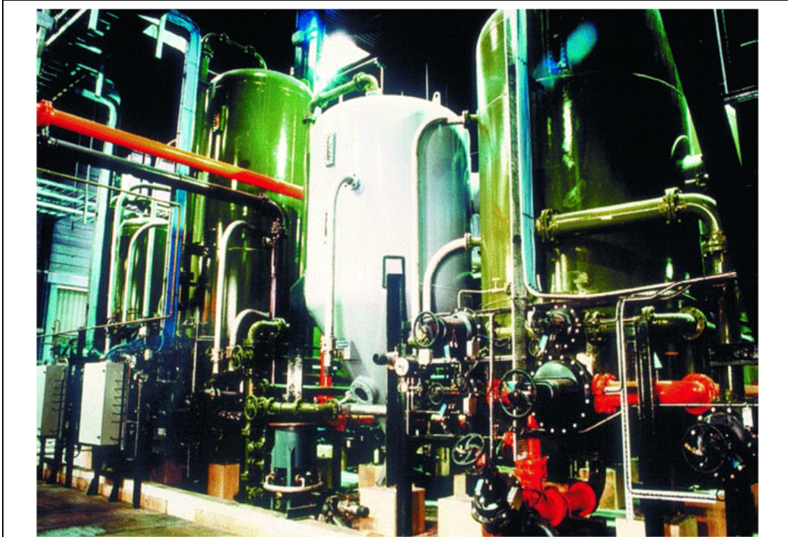
Figure 3.- Ion exchange system for boilers water supply. Dégremont Upflow double line system. Flow: 2 \times 48 m 3 /h. (Dégremont, 2001)
