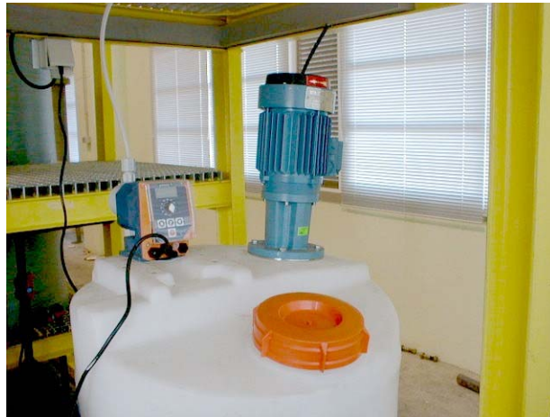
Figure 14 Solenoid pump installed on the dosing tank.
