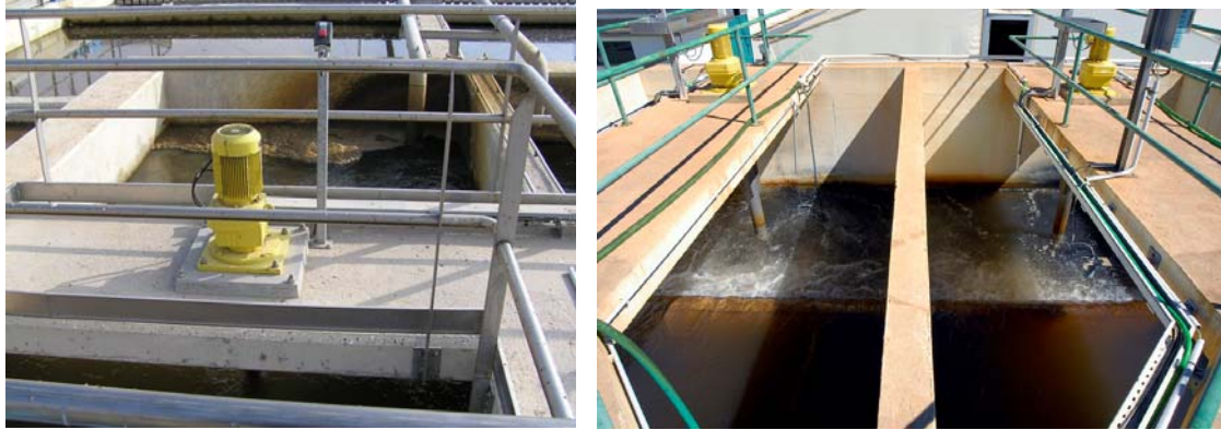
Figure 4 Engines for mixing in coagulation tanks.
