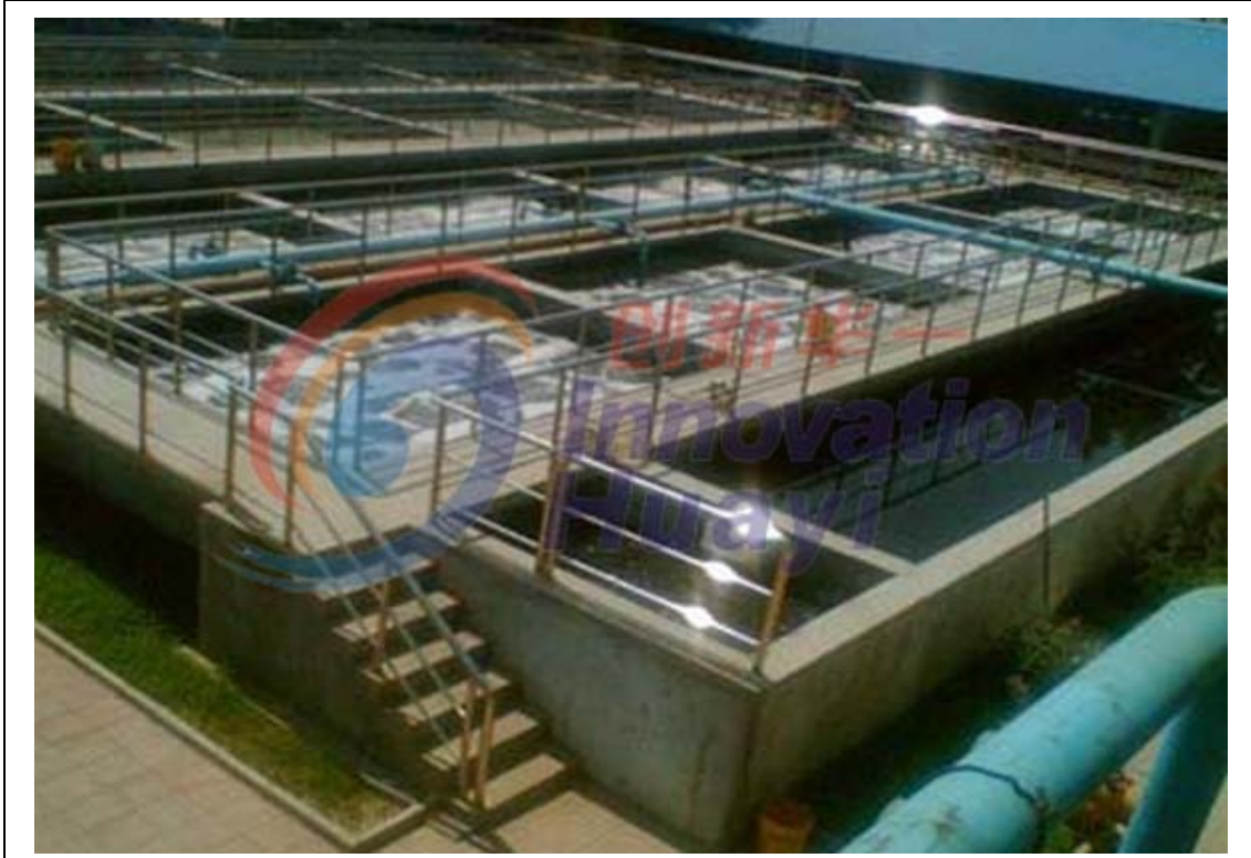
Figure 3.- Aerated biofilter system of technology Biocarbone
