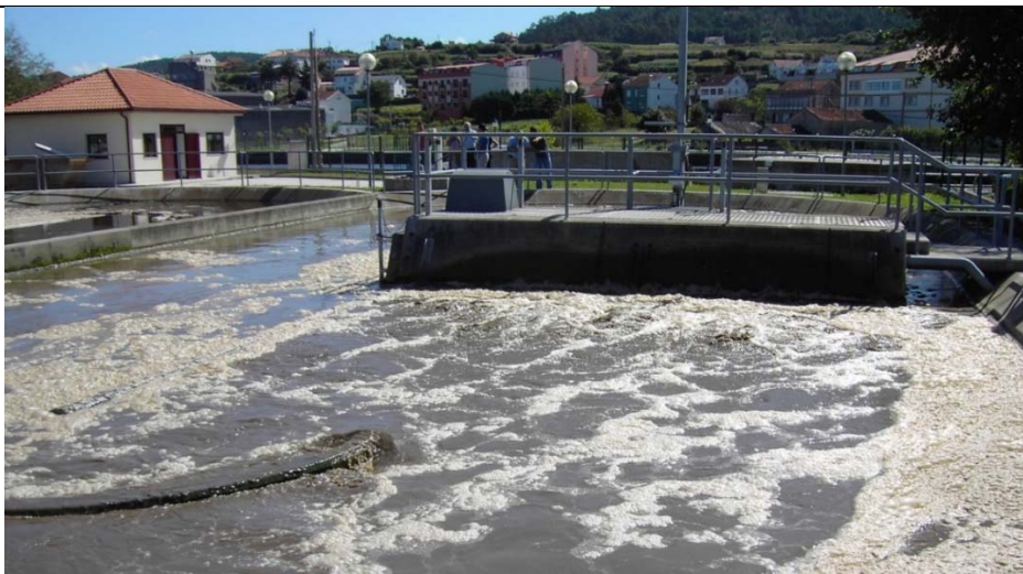
Figure 5 Activated sludge reactor (oxidation ditch technology). Municipal WWTP at Canduas (Spain) .
