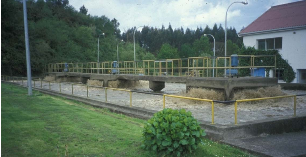
Figure 3 Activated sludge reactor. Industrial ETP at Bergondo (Spain).
